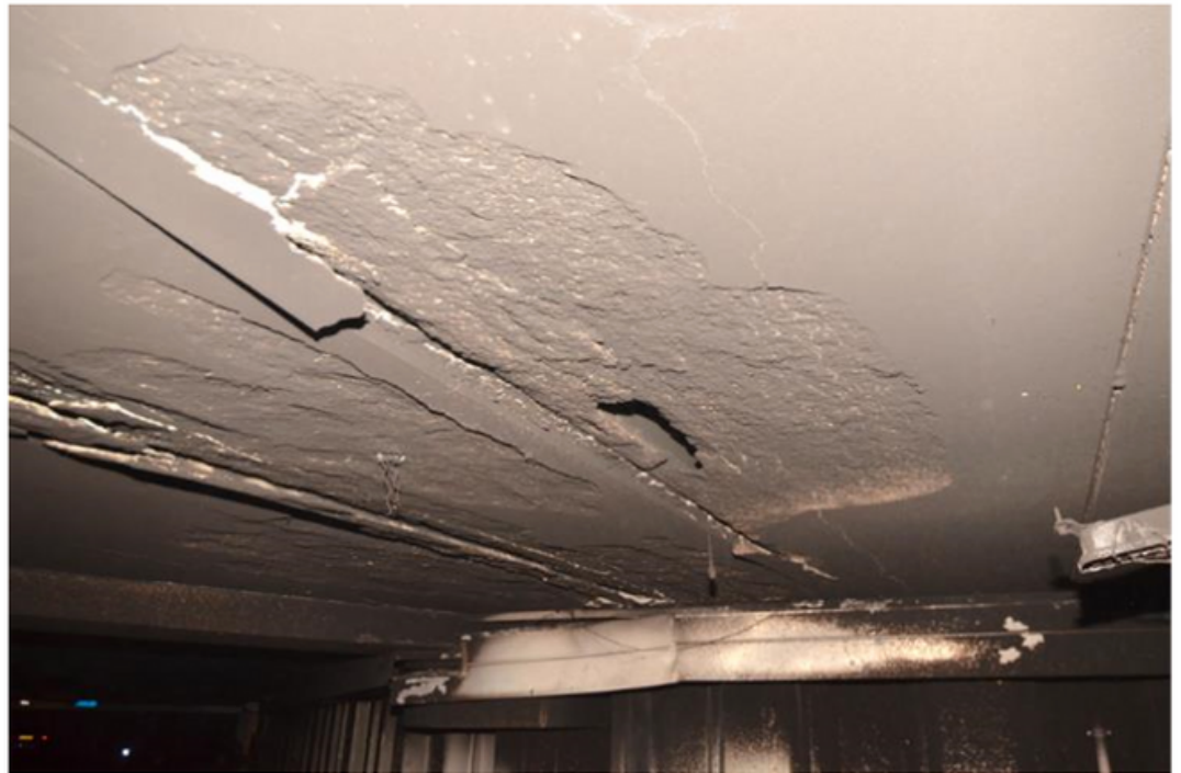
Ceiling spalling above Hyundai Ioniq BEV
