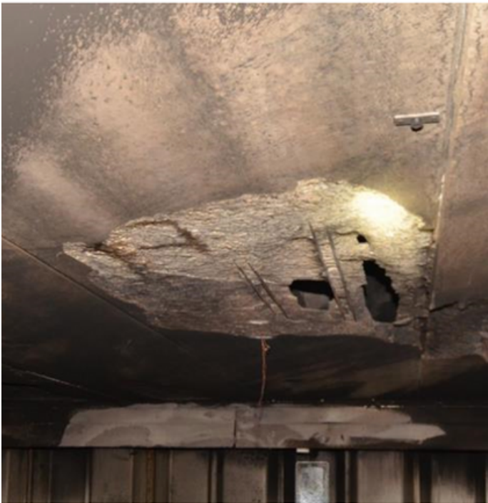
Ceiling spalling above Citroen C3 ICEV
