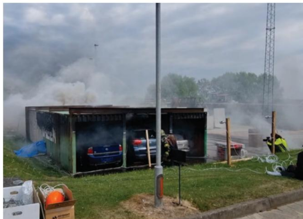
Photo 2: The fire in the battery pack is strong and has started to spread to the cabin.
