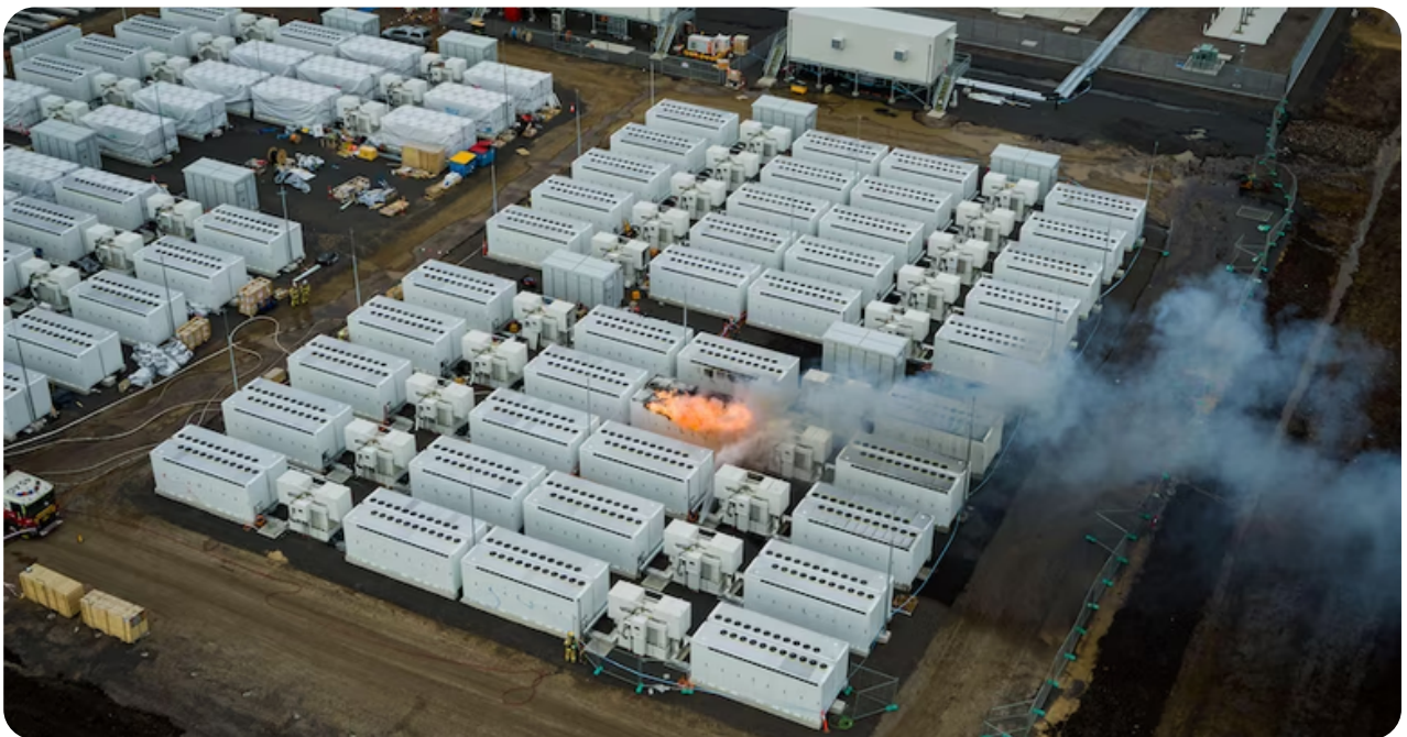
A fire in one of the Tesla Megapacks at the Victorian Big Battery during construction. The incident required a significant emergency response and burnt for over 3 days. Ref: Wong, L. 2021
