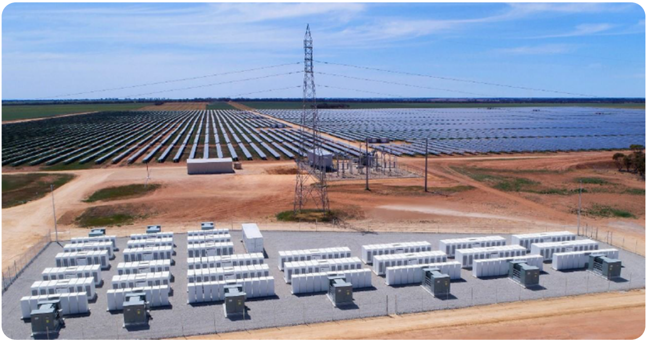
The Gannawarra energy project combines a 25MW / 50MWh BESS with a 50MW solar installation. The AAA is advocating for airports to adopt such installations. Ref: Edify, 2021.
