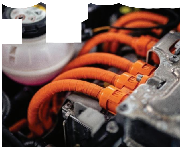
Cables with high voltage will most often be colored orange, as here in the engine compartment
